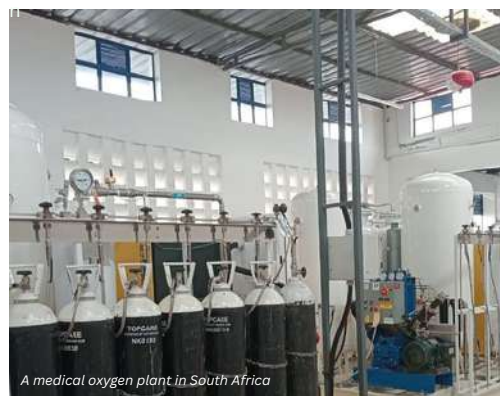
A medical oxygen plant in South Africa
